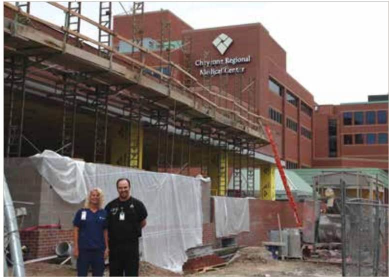
A new and better ED is coming to Cheyenne Regional! Tracy Garcia, Clinical Director for Trauma and Emergency Services stands in the construction zone with Dr. Dan Surdam, Medical Director of the ED.
